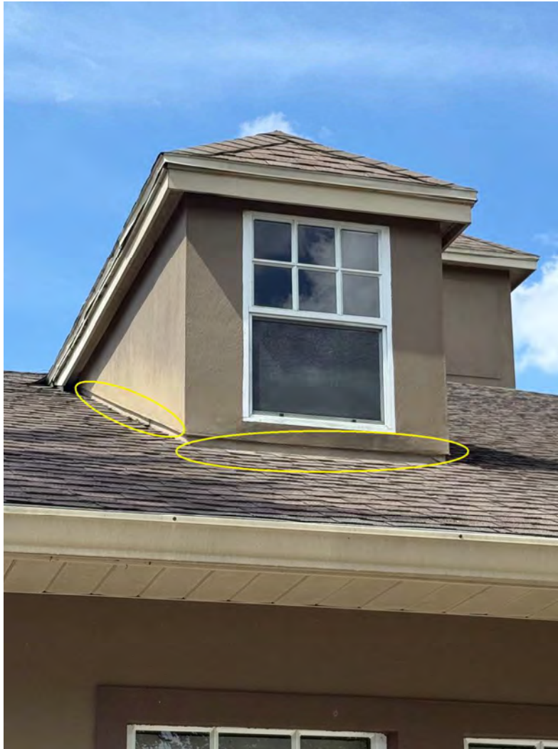
Photo 2 - Dormer / Wall Flashing Condition
